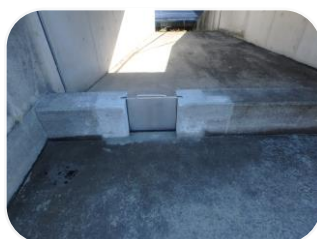
(洪水吐切欠き・北脇新池)
